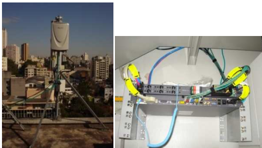
Fig. 4 – RRU (left-side); BBU and DC box (right-side).
