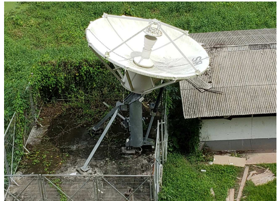
Fig. 2. 3 axes antenna installed in the Guamá STP.
